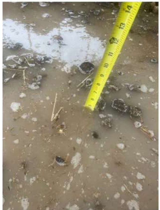
Standing water inside manure shed
