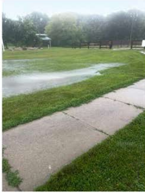
Water ponding around building
