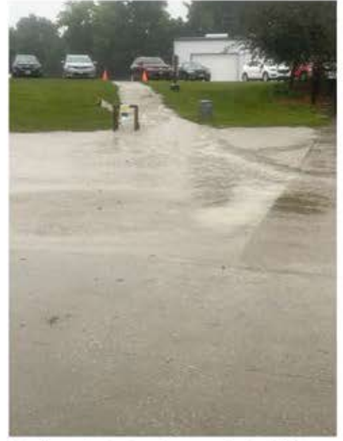
Water draining towards building
